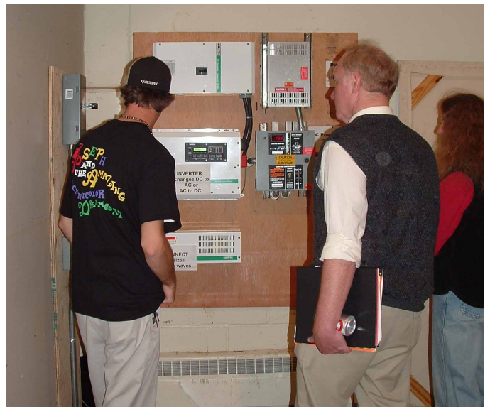
CDDHS Student Leader demonstrates the control panel for the Green Power Project, including metering equipment, inverter and “grid tie” system
